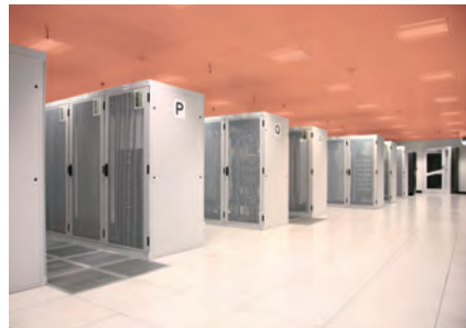
Ceiling protection at Data center
