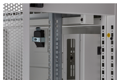
High-density vertical cable management
